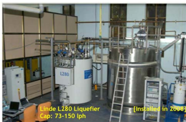
Figure 1. Linde L280 Helium plant at LTF.
