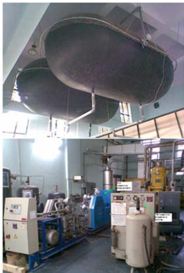
Figure 7. Helium gasbag & high pressure compressor.
