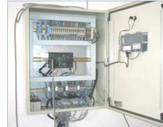
Fig. 4. Fiberglass Electrical Enclosure.
