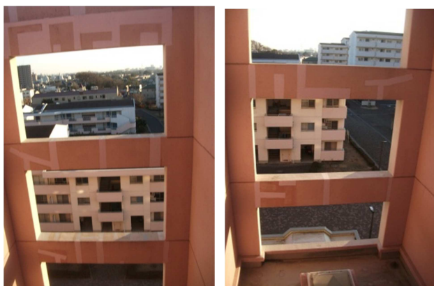
Figure 16. Back-Side of Horizontal Beams [Cracks propagated at white band portions before the epoxy resin was applied. (Photographed on 13 February 2013.)].
