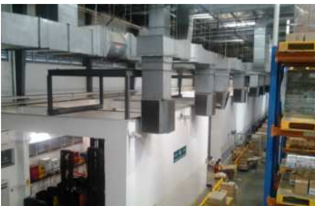
Figure 2. Mechanical Ventilation Return Air intake.
