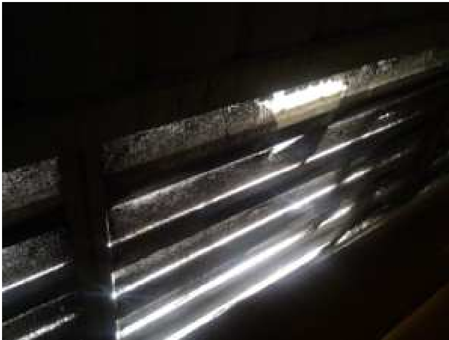
Figure 1. Insulation on Air Grills.
